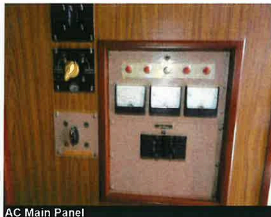
AC Main Panel
